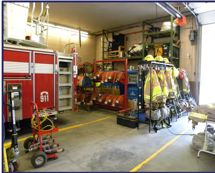
Storage for hose and bunker gear. Note the SCBA Refill Station behind the hose.
