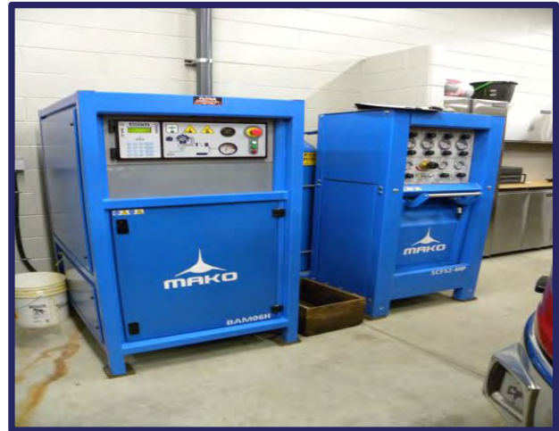
SCBA Bottle Refill Station Maintenance
