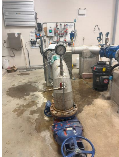
FIGURE 18 - INTERIOR OF BROWNLEY PUMPHOUSE SITE
