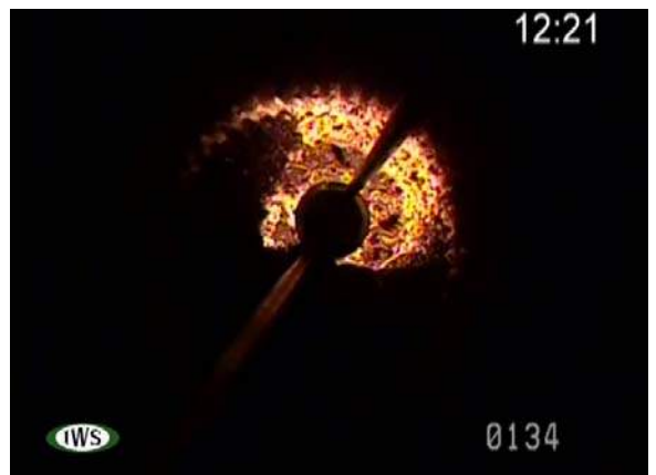
Partial blockage near bottom at 134 feet
