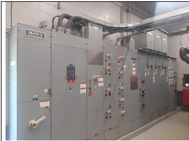
FIGURE 8 - COMPLETE MCC PANEL AT MILL STEET SITE (NORTHWEST)
