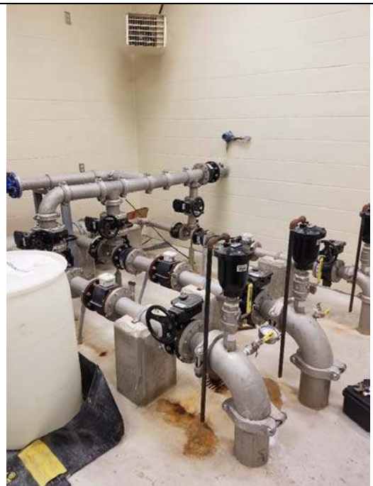
Treatment Plant piping with line to waste through wall
