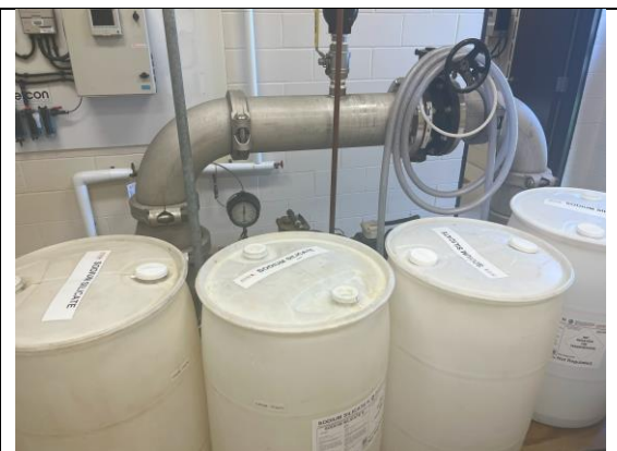
FIGURE 30 - CHEMICAL STORAGE TOTES INSIDE CHEMICAL STORAGE BUILDING
