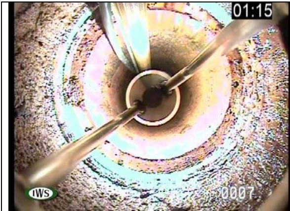
Pitless seat in poor condition at 7 ft
