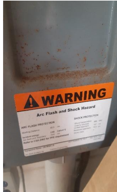
FIGURE 41 - INTERIOR OF ELECTRICAL PANEL SHOWING SIGNS OF CORROSION
