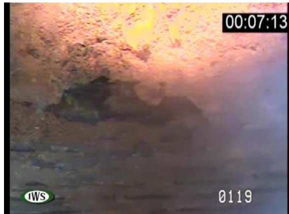
Casing corrosion at K-Packer at 119 ft
