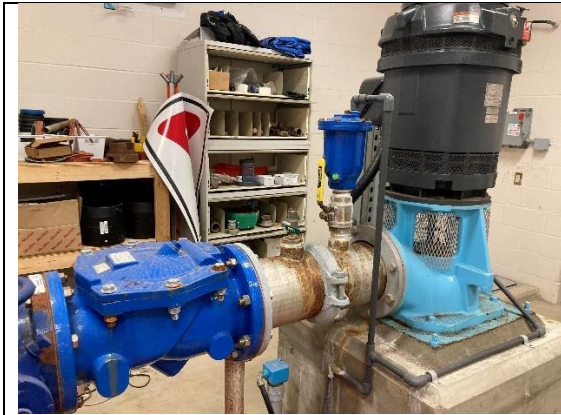
FIGURE 27 - PROCESSING PIPING INSIDE OF PUMPHOUSE (EAST)
