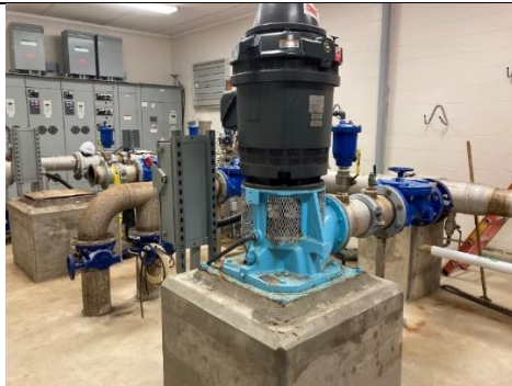
FIGURE 20 - INTERIOR OF BROWNLEY PUMPHOUSE SITE
