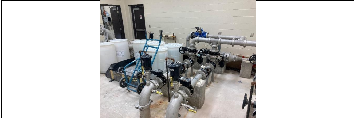
FIGURE 31 - PROCESSING PIPING AND CHEMICAL STORAGE TOTES IN CHEMICAL STORAGE BUILDING
