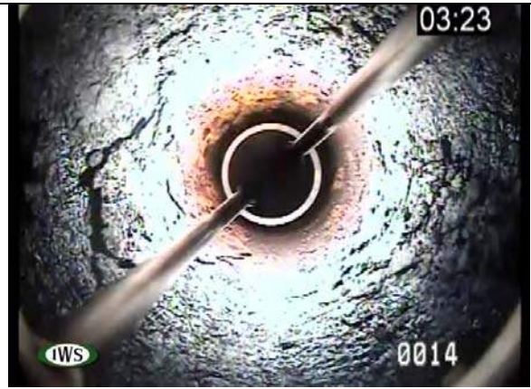
Casing in poor condition at 14 ft
