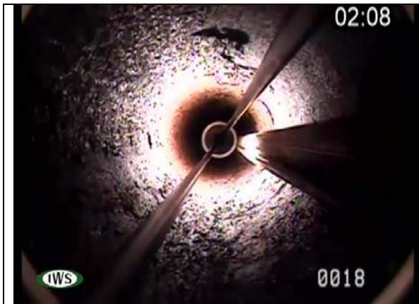
Loose corrosion scale at 18 ft
