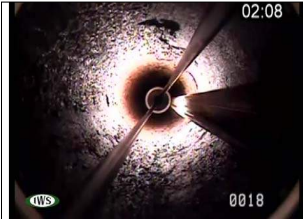
Loose corrosion scale at 18 ft
