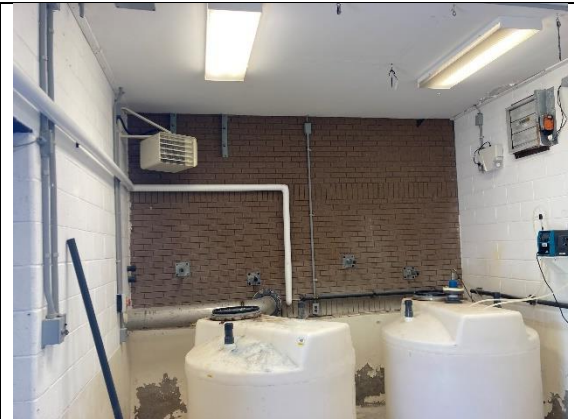
FIGURE 11 - UNIT HEATER AND MOTORIZED LOUVRE IN CHEMICAL STORAGE
