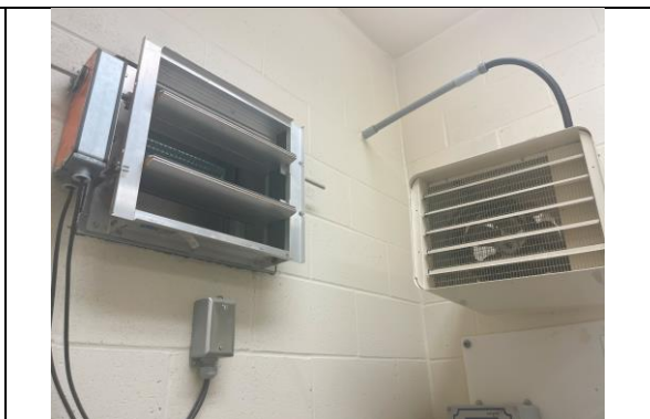
FIGURE 26 - UNIT HEATER, MOTORIZED LOUVRE AND EXHAUST FAN IN CHEMICAL STORAGE BUILDING SITE
