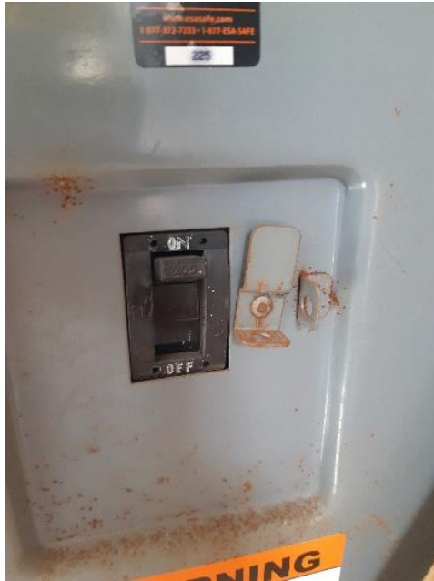
FIGURE 40 - INTERIOR OF ELECTRICAL PANEL SHOWING SIGNS OF CORROSION
