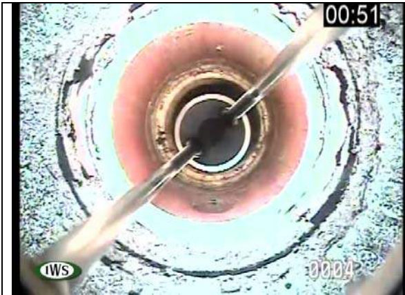
Corrosion of upper spool on pitless at 4 ft
