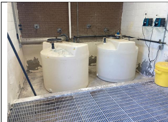
FIGURE 12 - CHEMICAL STORAGE TOTES INSIDE OF CHEMICAL STORAGE (NORTH) SITE
