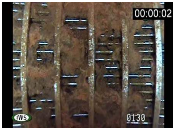
Horizontal view of deposits on screen at 130 feet
