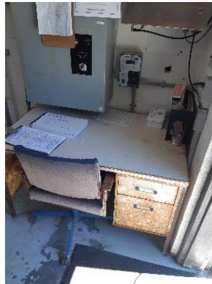
FIGURE 43 - SPACE IN FRONT OF MAIN BREAKER/VFD/ATS, SHOWS LACK OF SPACE (2)
