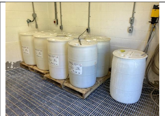
FIGURE 13 - CHEMICAL STORAGE TOTES INSIDE OF CHEMICAL STORAGE (SOUTH) SITE
