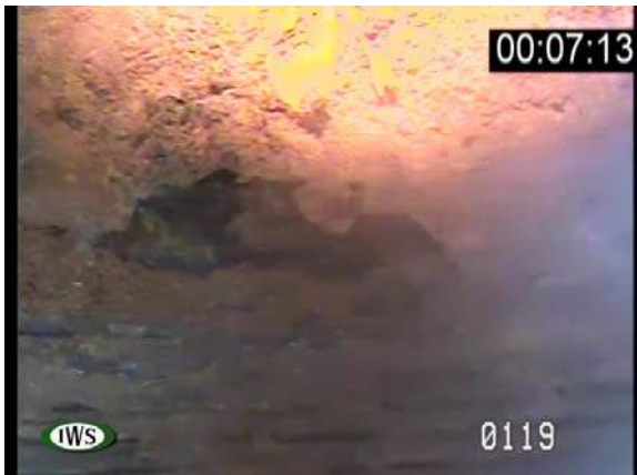
Casing corrosion at K-Packer at 119 ft
