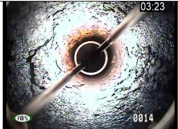
Casing in poor condition at 14 ft
