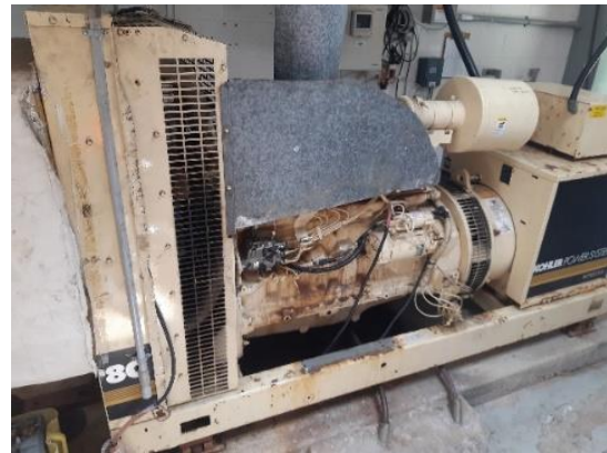
FIGURE 45 - CURRENT CONDITION OF DIESEL GENERATOR
