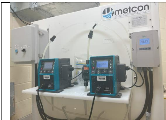
FIGURE 29 - CHEMICAL DOSING PUMPS INSIDE CHEMICAL STORAGE BUILDING
