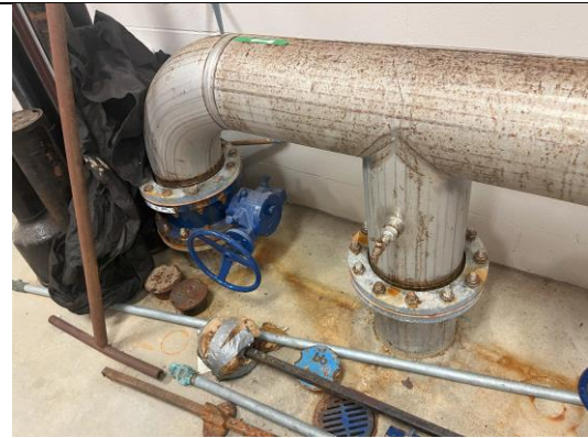
FIGURE 28 - PROCESSING PIPING INSIDE OF PUMPHOUSE (WEST)
