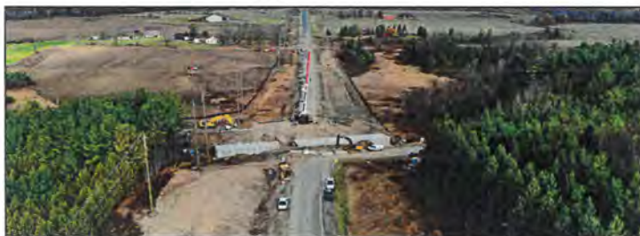
The County is investing $64M in capital project expenditures to enhance road networks across Simcoe County, with major projects continuing on County Road 22, County Road 21 (Innisfil Beach Road), County Road 4 (image above).
